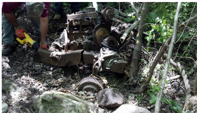
Frank uses a battery-powered hacksaw to cut up the vehicle's frame into manageable pieces.
