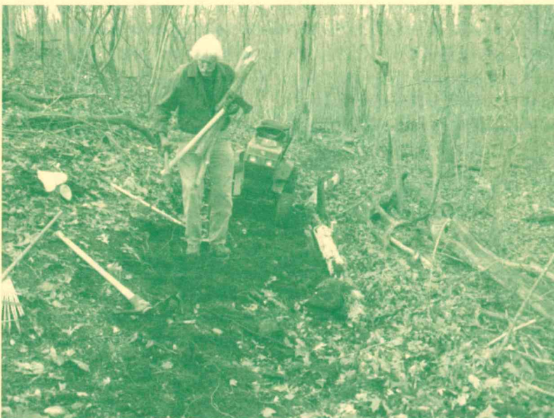
Mac Turner works on establishing the new trail through the Henne Preserve.
