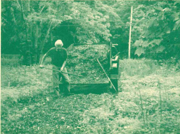
Mac Turner installs the path from Clarks Falls Road to the footbridge over the brook.
